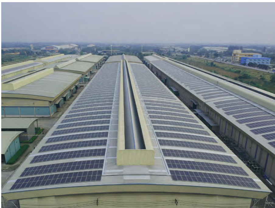
Solar PV Rooftop 2.5 MW
