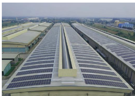
Solar PV Rooftop 2.5 MW
