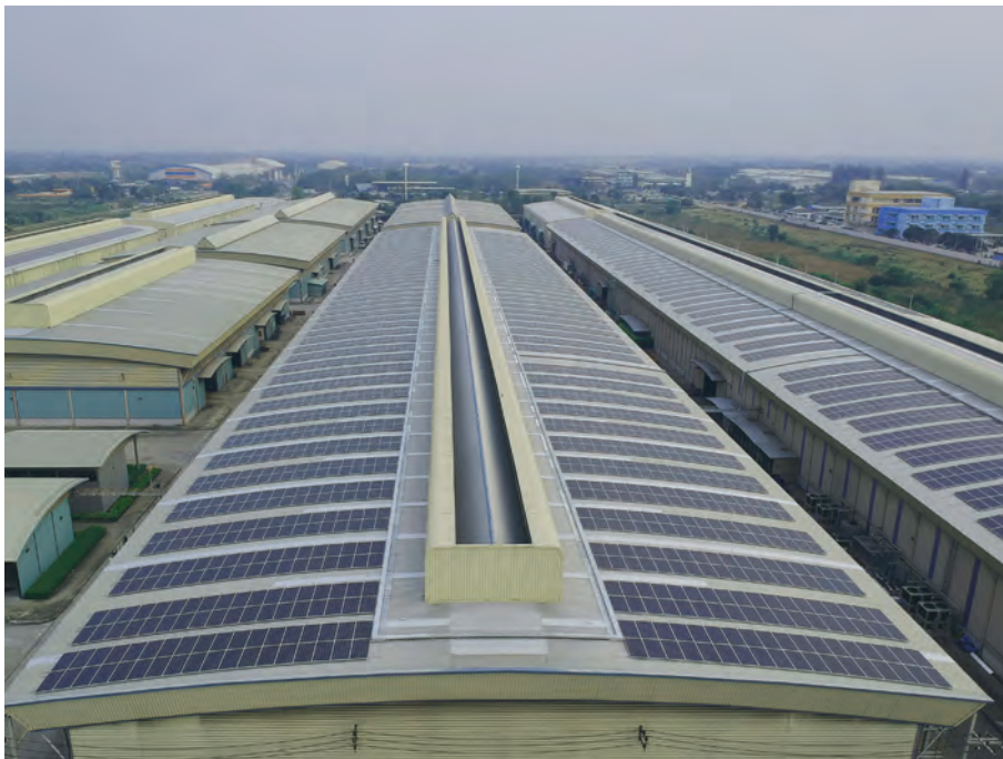
Solar PV Rooftop 2.5 MW
