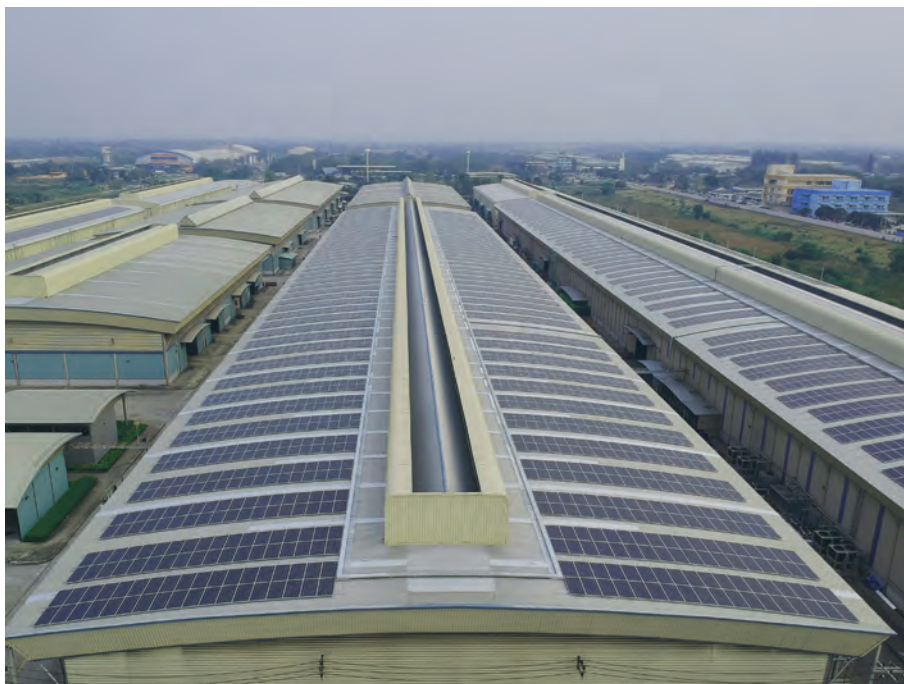
Solar PV Rooftop 2.5 MW
